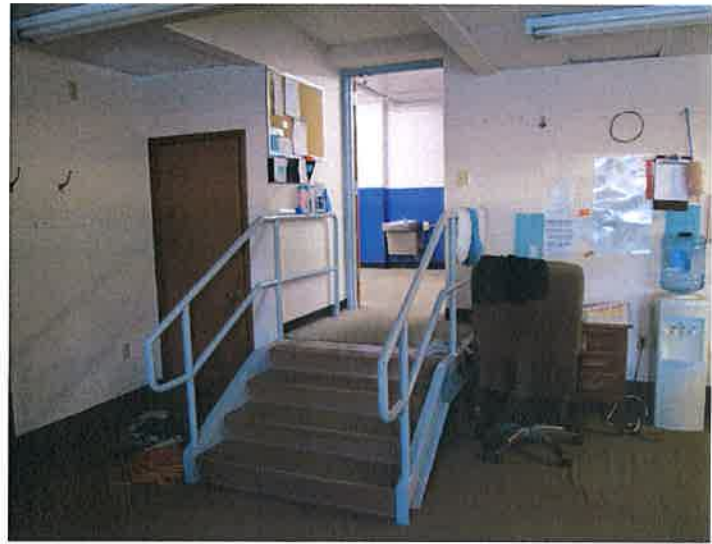
Custodial office is not handicap accessible
