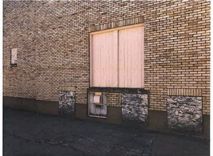
Many windows are removed and have a plywood infill
