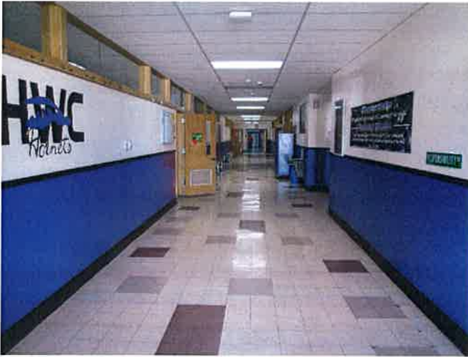
Corridors are not fire rated - cannot have glazing at corridor walls and doors cannot have louvers if the building isn't sprinklered
