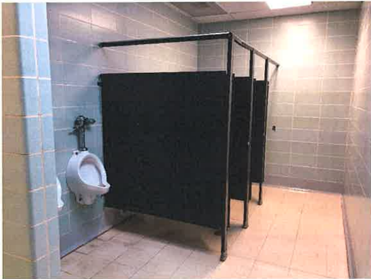
Restroom fixtures and finishes past their life expectancy
