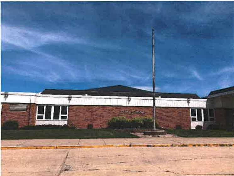
Downspouts do not extend down to the ground
