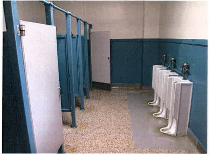
Urinals cannot drain at floor level – restrooms are not handicap accessible
