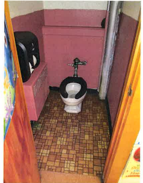
Toilets do not meet ADA clearance requirements
