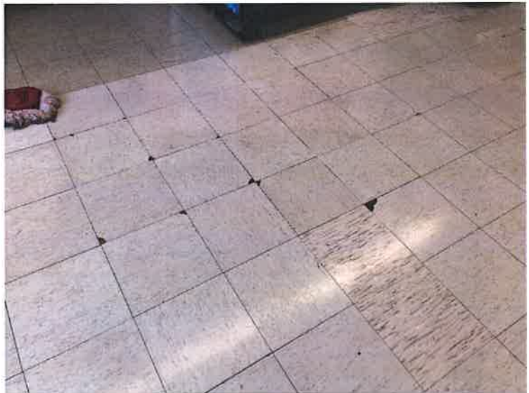
VCT flooring needs to be replaced in various locations
