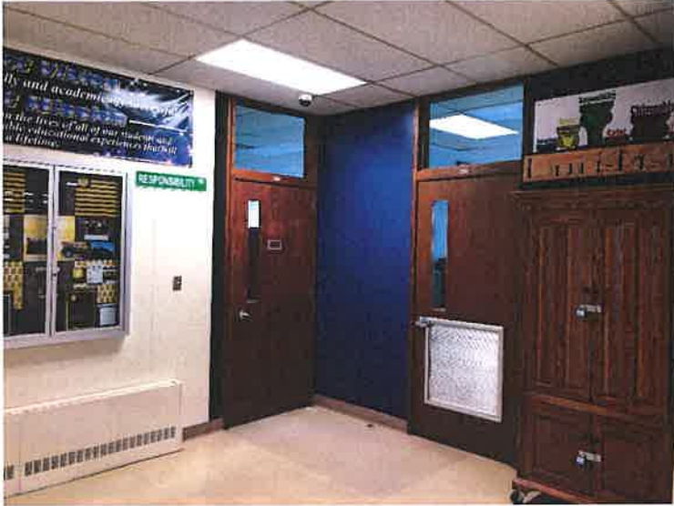
Cannot have louvers in doors or glazing in doors without a sprinkler system
