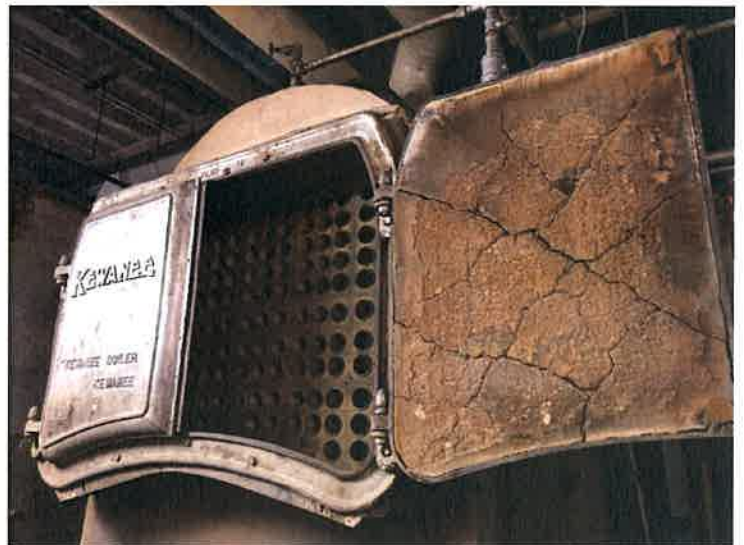
Coal boiler is outdated
