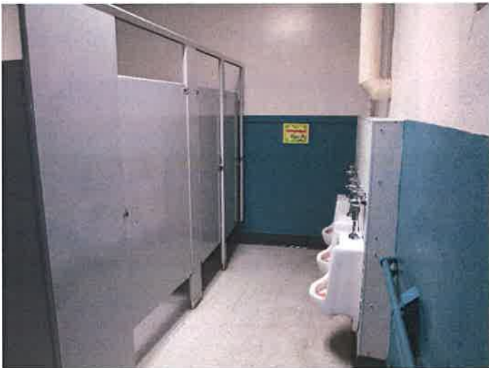
Restrooms do not meet ADA clearances
