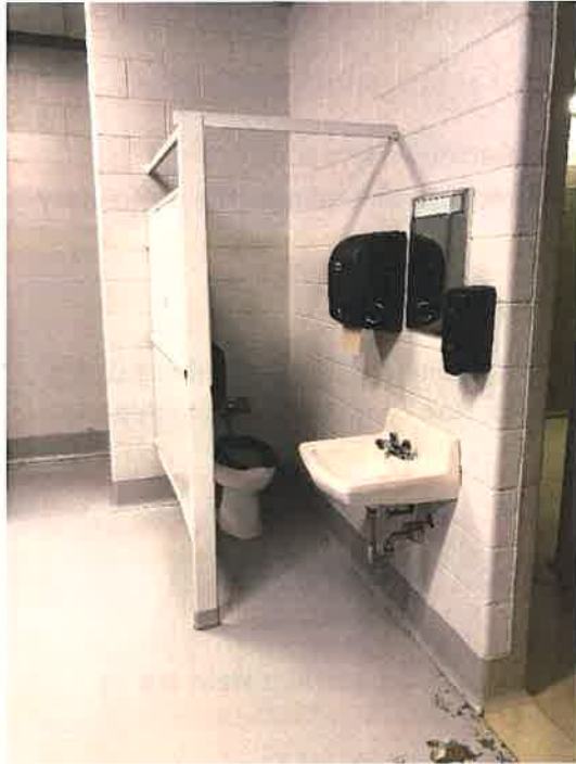
In the locker room the toilet stall does not meet handicap accessibility and floor paint needs to be repaired
