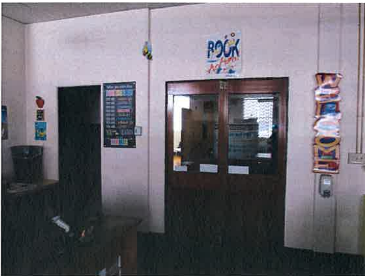
Doors do not have accessible hardware and cannot have top and bottom locks
