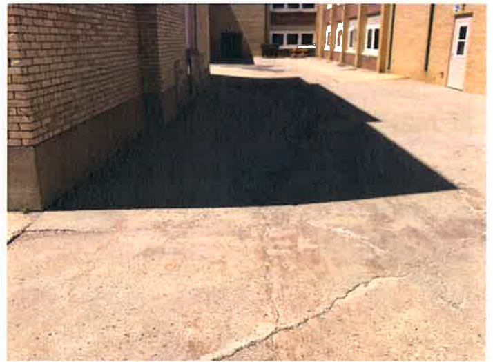
Back courtyard between the building additions is sinking and causing storm sewer collapse
