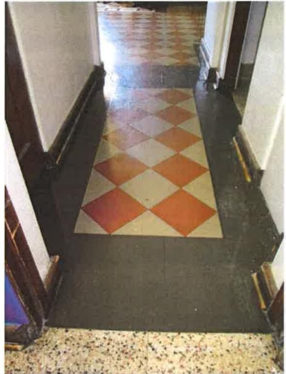
Flooring and wood trim are past their expected useful life
