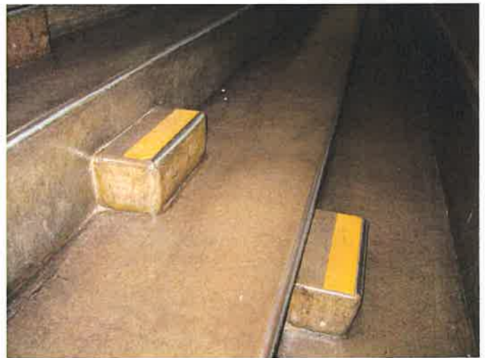
Stadia stairs are missing intermediate handrails and are too narrow
