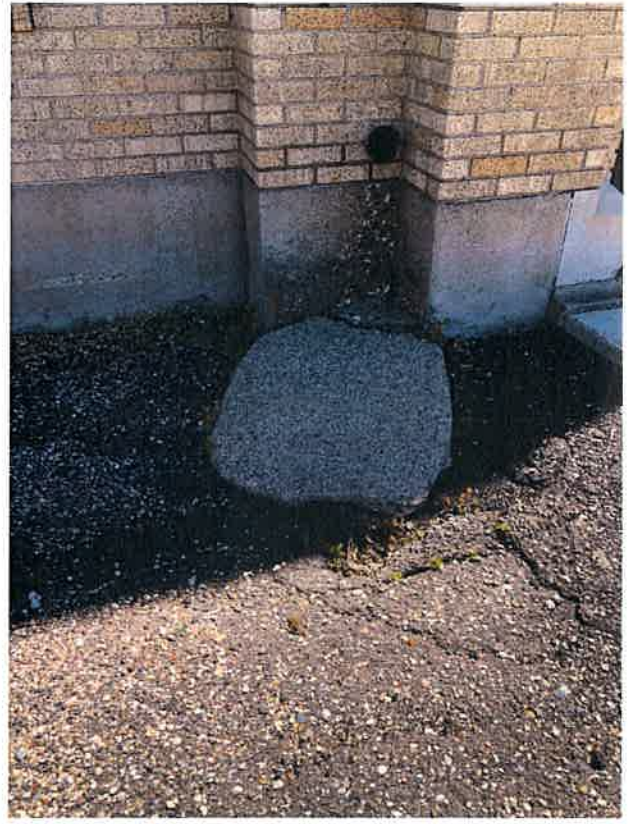
Drainage freezing and thawing damage throughout the site
