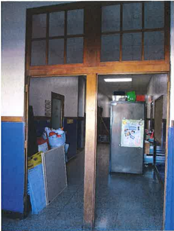
Vestibule doors missing
