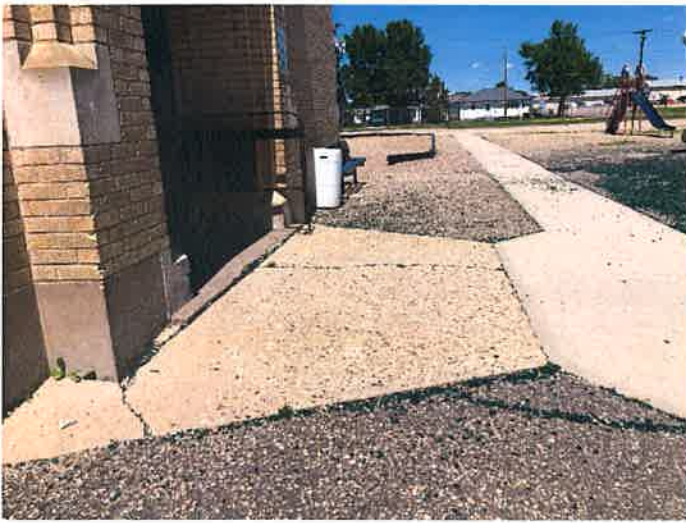
Sidewalk and brick deterioration
