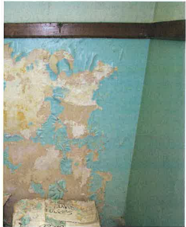
Storage under the stage has water infiltration and potential mold
