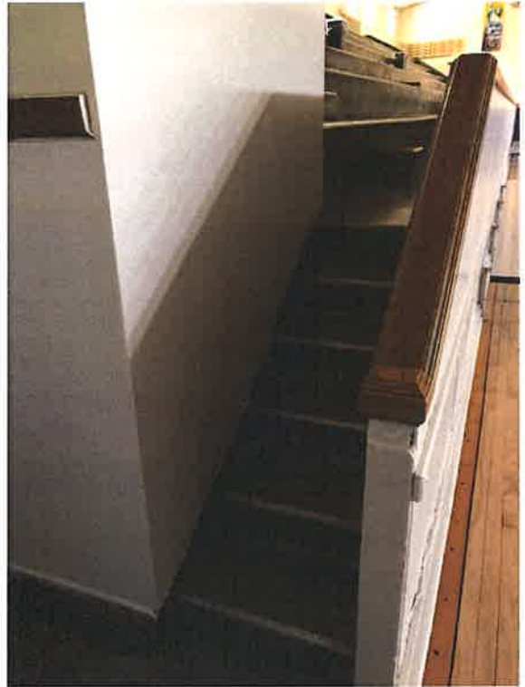
Stadia stairs are too narrow, are missing handrails, and the guard railing is too low
