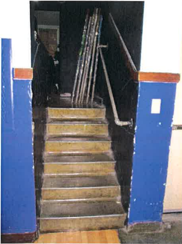
The stage is not handicap accessible – the stair handrail is not ADA compliant
