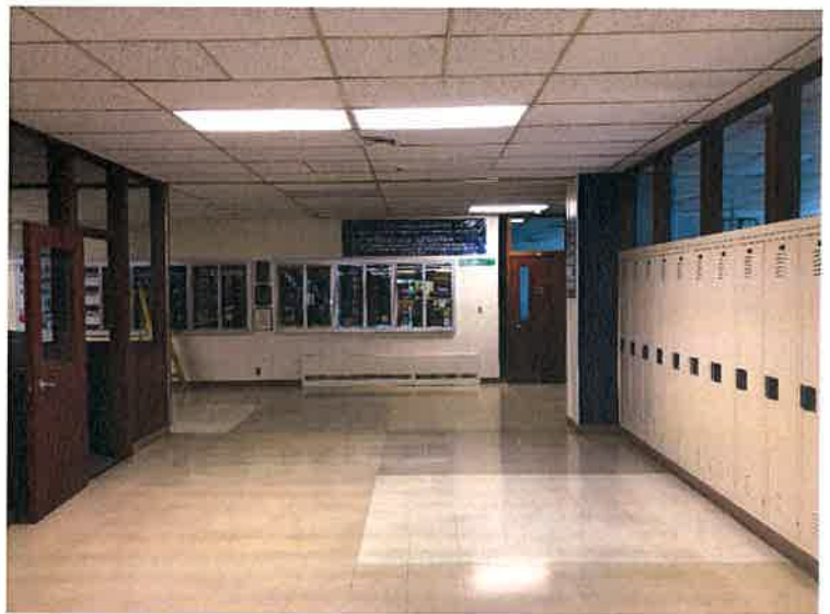
Corridors are not fire rated – cannot have glazing at corridor walls without sprinkler system
