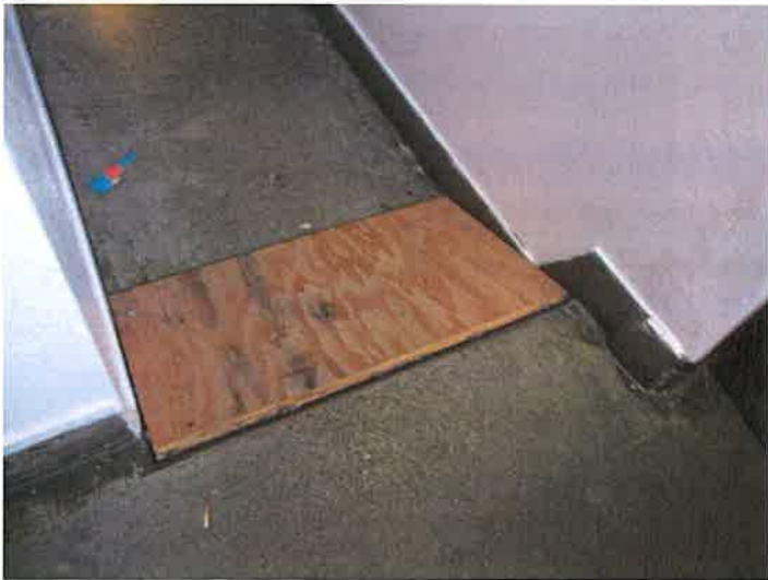
Makeshift wooden ramp into the locker rooms is not ADA compliant
