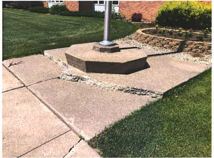
Pavement/sidewalk is cracked and heaved
