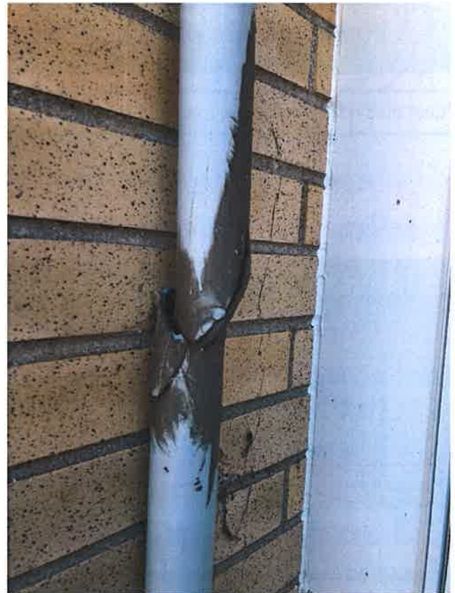
Downspouts are damaged
