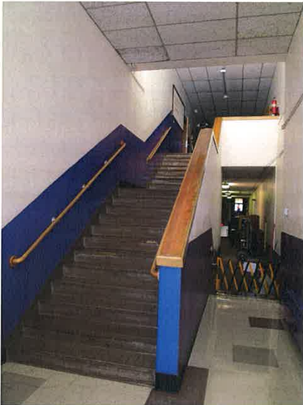
Corridor narrows next to stairs and stair handrails do not extend 1' 0" past the bottom tread
