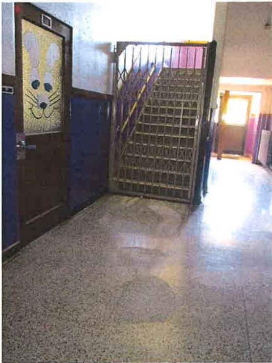
Stairs do not lead directly outside and cannot be blocked with movable gate
