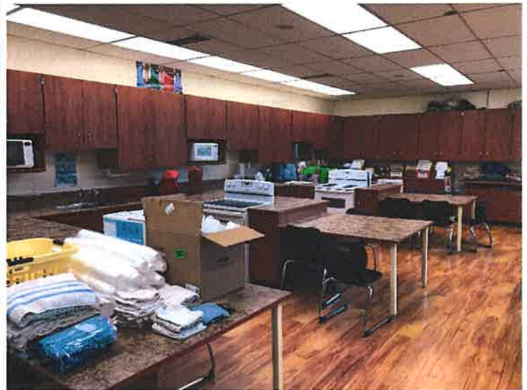
FACS area lacking accessible casework and fixtures
