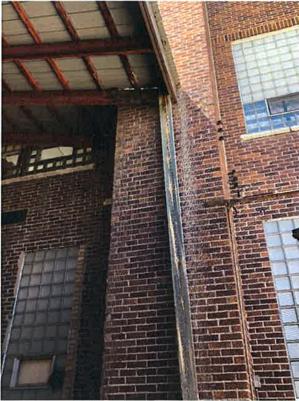
Coal shed is in poor/unstable condition
