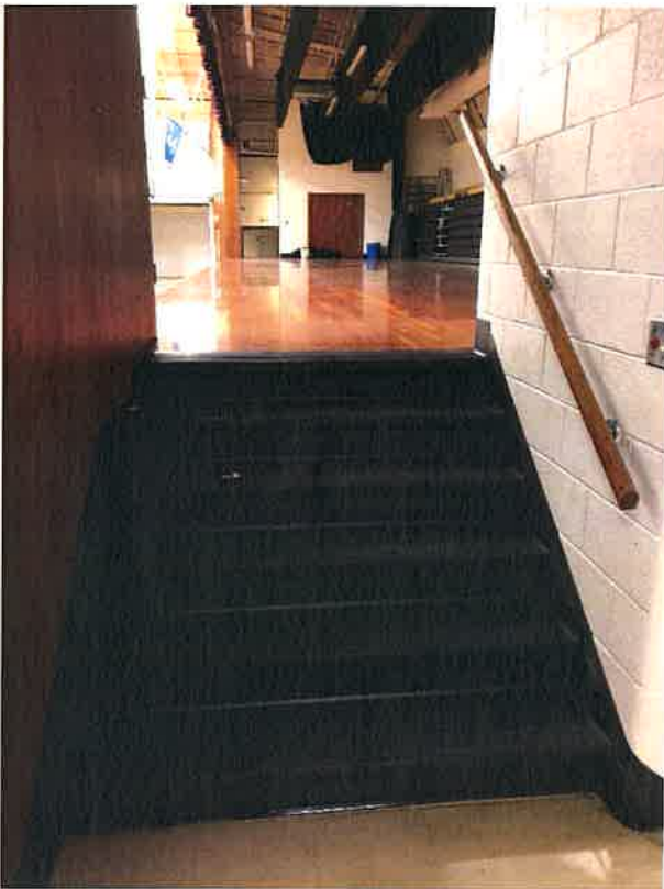
Stage is not handicap accessible – missing a handrail
