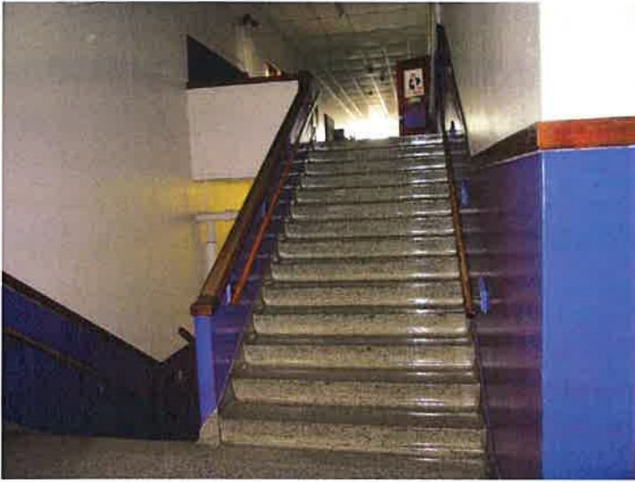
The stairs are not enclosed/don't lead directly outside and the guard rails are too low
