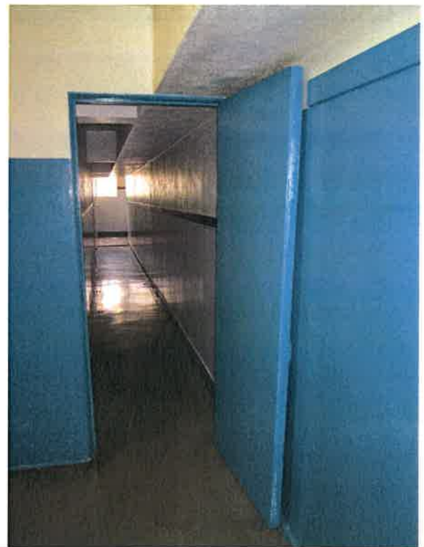
Corridor to the locker rooms is too narrow and it lacks head clearance
