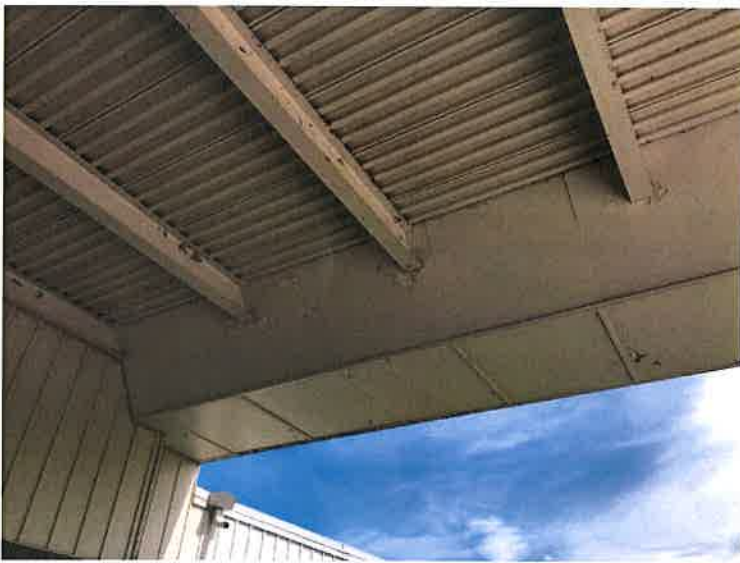
Front entrance canopy paint peeling
